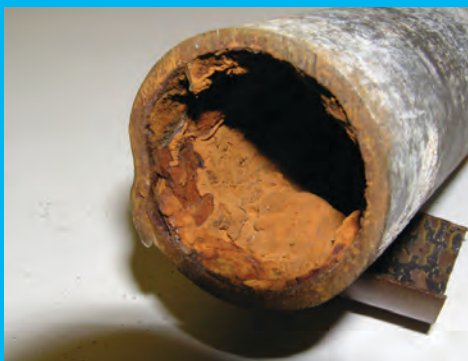
A pipe exposed to corrosion.
